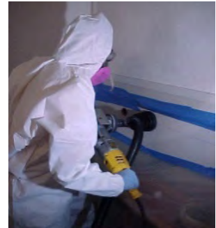
FIG. E-10: HEPA SHROUDED POWER TOOL
